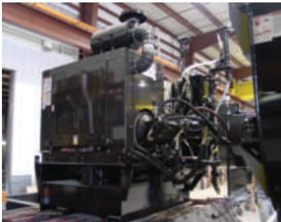
QSB6.7 Cummins Power Unit powering a hydraulic pump.
