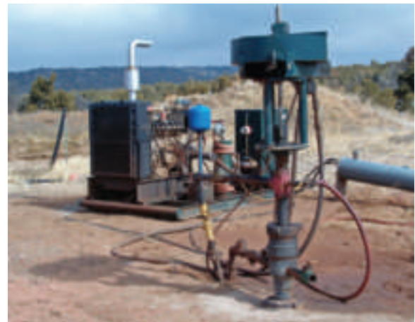
G8.3 Natural Gas Cummins Power Unit in a gas compression application.
